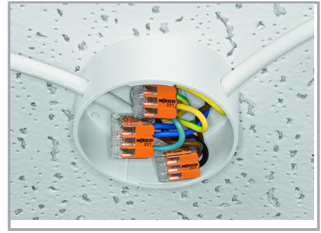
Lighting distribution in a ceiling canopy
